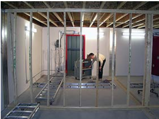
One of the chambers in the new NRC-IRC flanking research facility.
